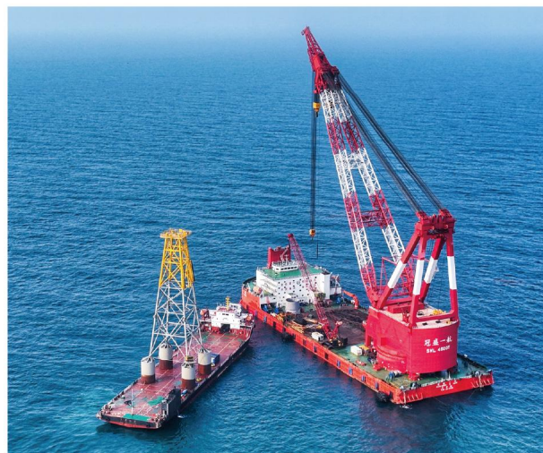
Zhangpu Offshore Wind Farm Met Mast, Fujian, China
