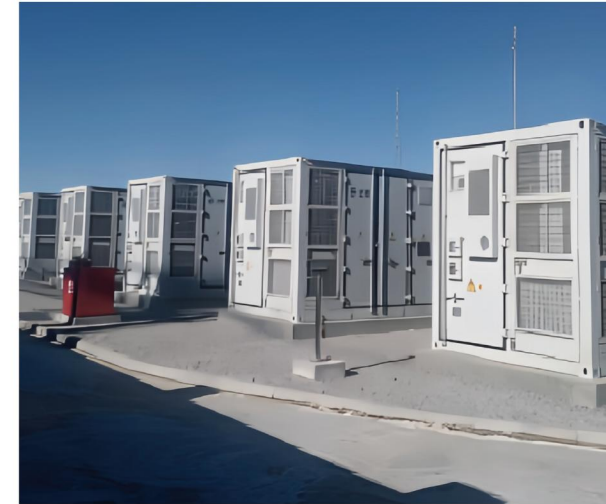
Guazhou 750MW/2100MWh Energy Storage Plant, Gansu, China
