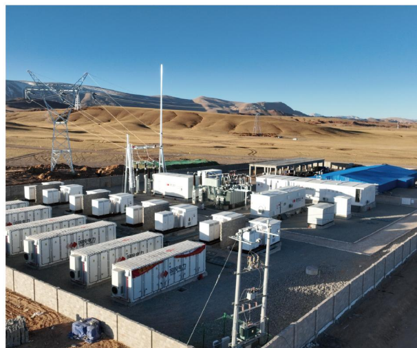
SDIC POWER NIMA 50MW Solar PV & Energy Storage Project, Xizang, China
