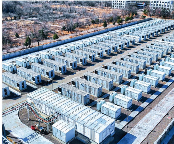
SG-CATL Huadian Datong 150MW/300MWh Energy Storage Plant, Shanxi, China
