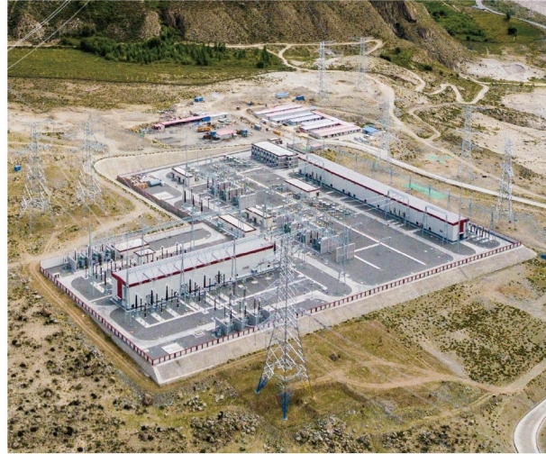
Yazhong 500kV Substation Project, Xizang, China
