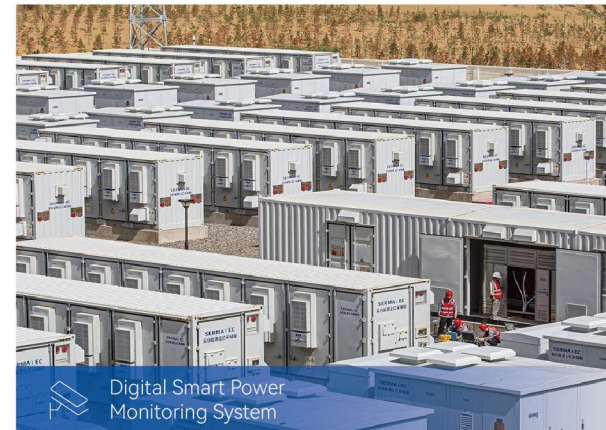
Mengxi Base Kubuqi Desert Solar PV Plant Project, No.1 Energy Storage Station (80MW/160MWh), Inner Mongolia, China
